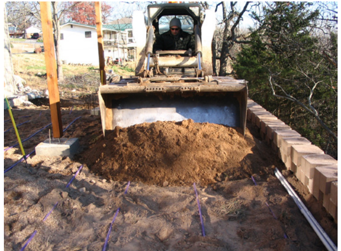
After laying the dripperline out in evenly-spaced rows, soil is laid over the tubing. NOTE: the operator is keeping the loader parallel to the tubing to minimize any shifting.
