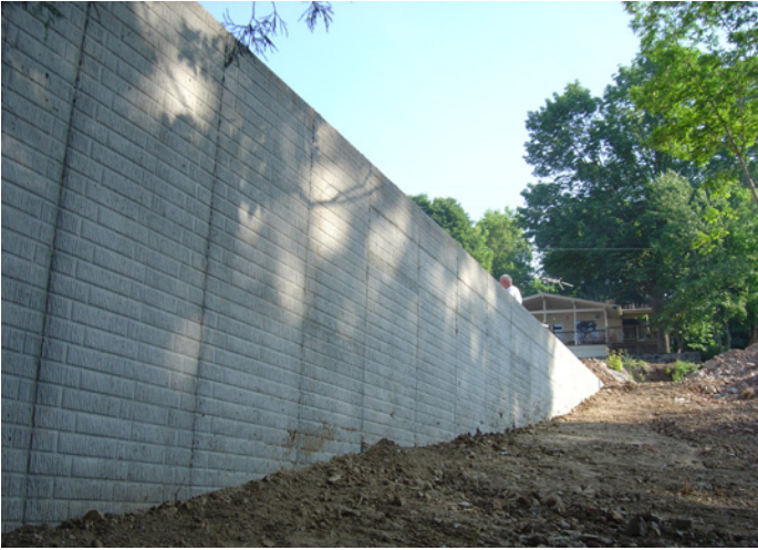
View of the retaining wall that was built to house the treatment system and much of the drip dispersal field.
