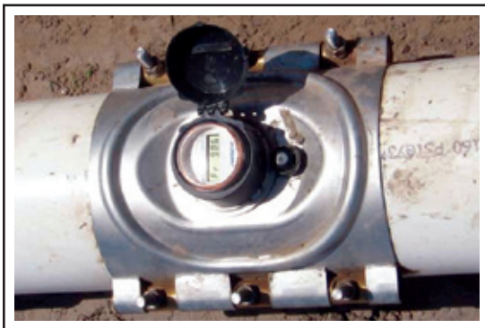
The above is an example of a saddle meter installed on a mainline.
